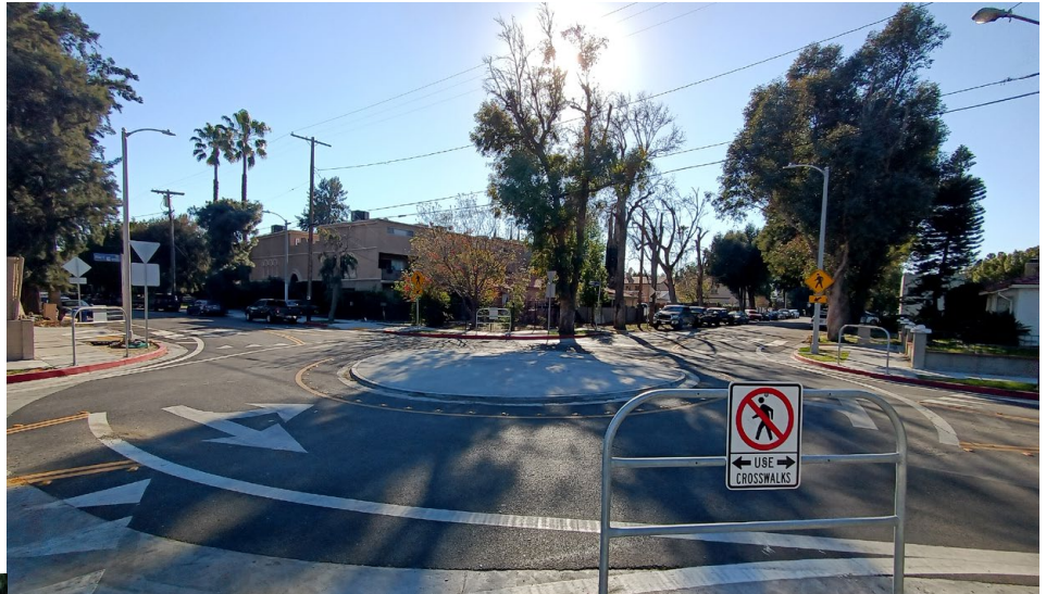
A new roundabout was constructed on the intersection of Hart Street and Baird Avenue.
