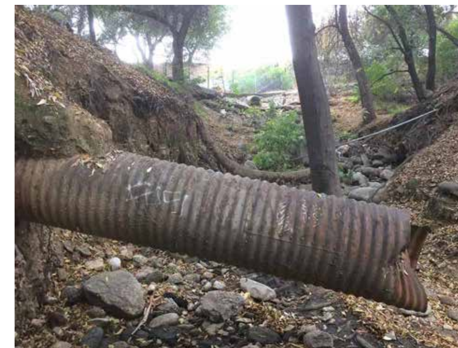
Figure 13. Before (with below): Degraded conditions along Berkshire Creek. Source: PSOMAS, 2019.
